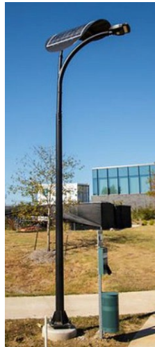
Figure 6H: Solar-Powered Light
