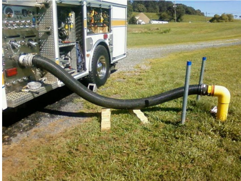
Figure 6. Example of what it will look like to attach fire truck to coupler
