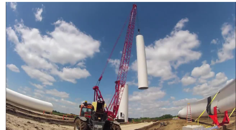
The hoisting of the mid-tower section to be installed. Source: MidAmerican Energy
