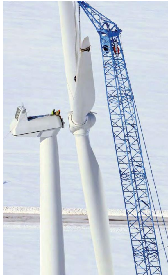
Assembling the hub with three wind turbine blades to the nacelle. Source: (WE Energies 2012)
