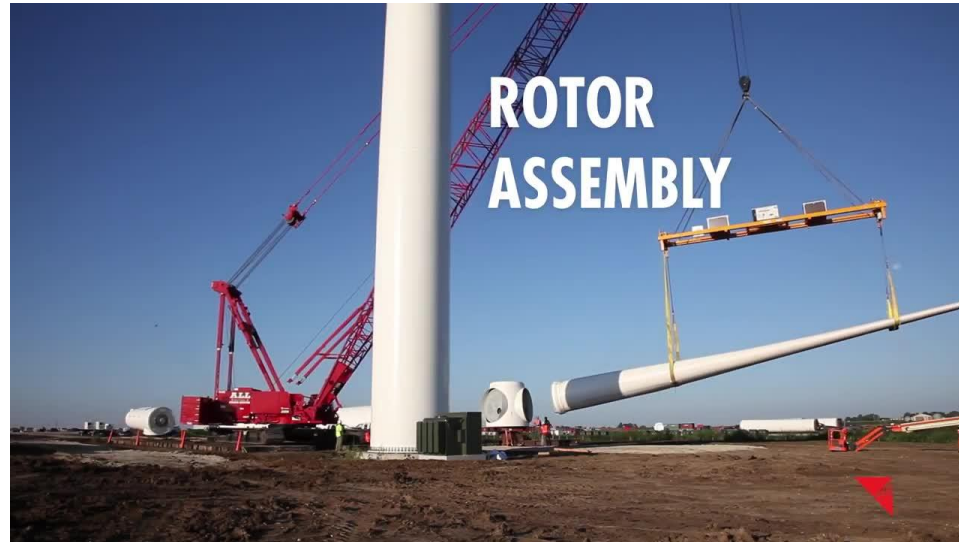
The assembly of the wind turbine rotor and blades with cranes. Source: MidAmerican Energy
