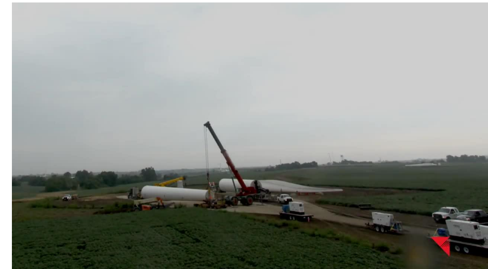
The delivery of the wind turbine components to the construction site. Source: MidAmerican Energy
