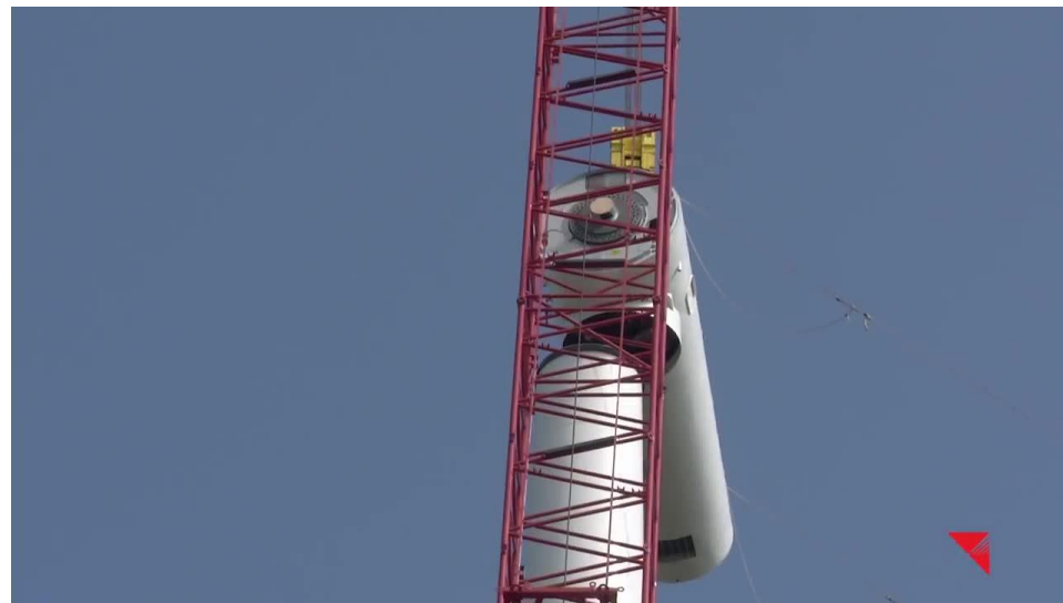
Hoisting the nacelle to the top of the wind turbine tower for installation. Source: MidAmerican Energy
