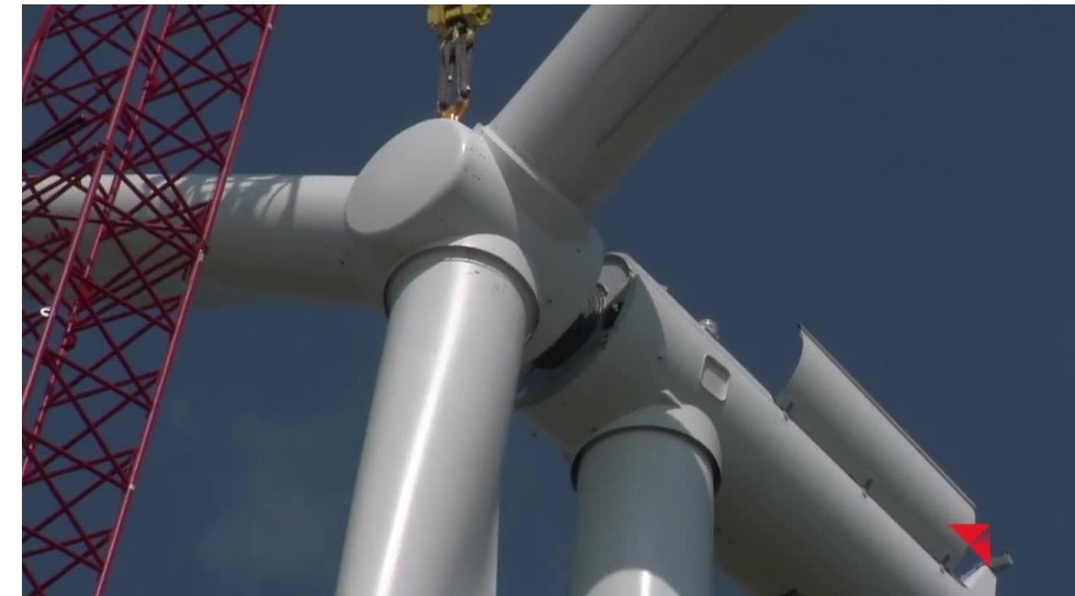
Installation of the rotor with attached blades to the nacelle. Source: MidAmerican Energy
