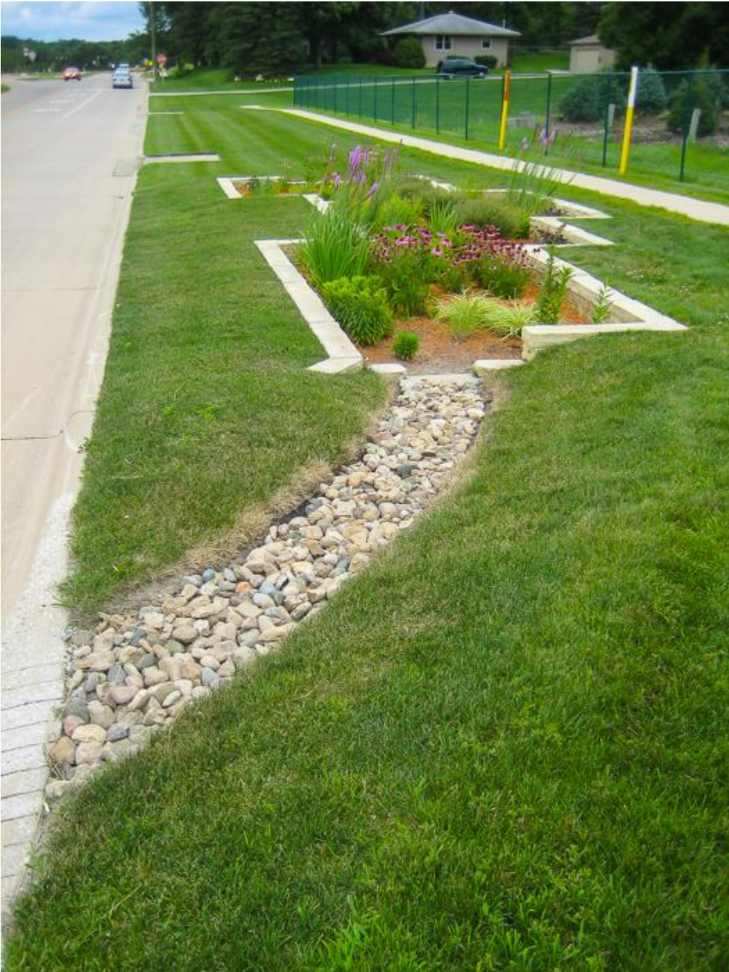
Figure 8.2 Pretreatment Rip Rap
