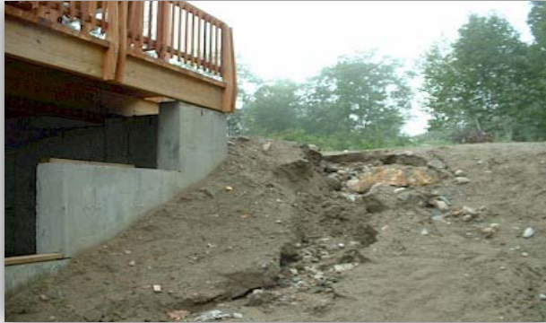
Figure 7: Erosion Caused by Stormwater Runoff ( http://www.state.me.us/dep/blwq/images2/erosion1a.jpg )
