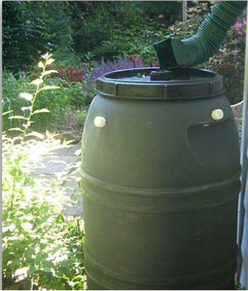
Figure 15: Down Spout into a Rain Barrel
