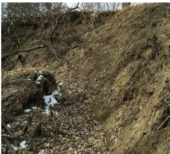
Figure 3a: Banks sliding into creek
