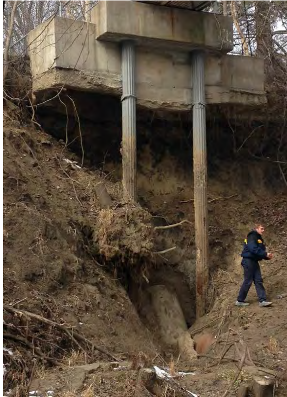
Figure 2: Extreme erosion at Clark Elementary pedestrian bridge
