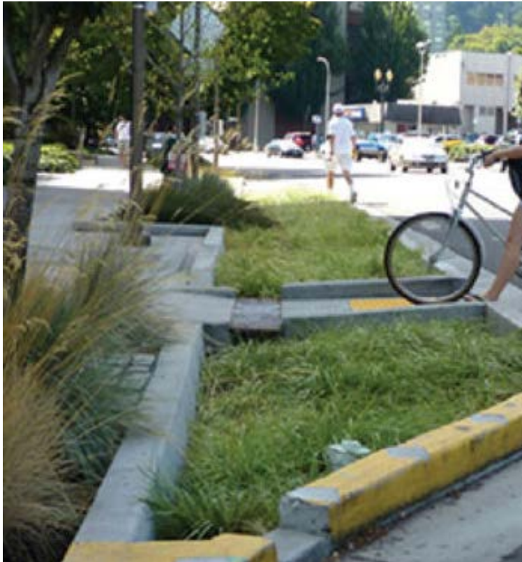
Figure C4. Steel plate in bump-out sidewalk allowing water to flow under the sidewalk.
