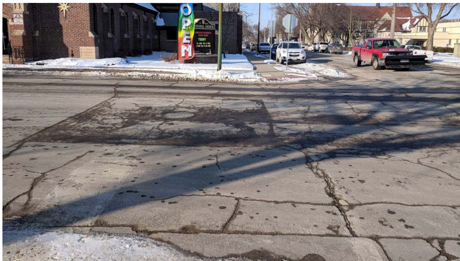
Figure 2. PCC pavements from utility work in poor condition
