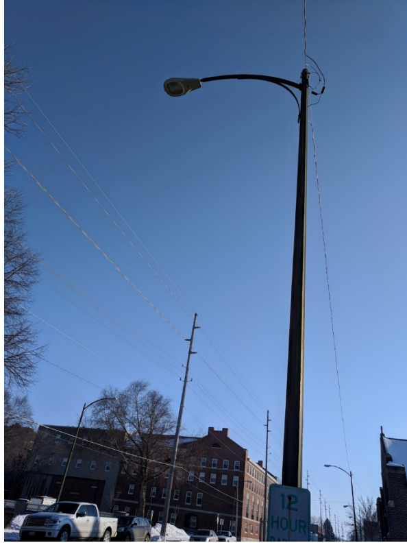
Figure 3. Existing street light along Pennsylvania Ave. showing above ground wiring
