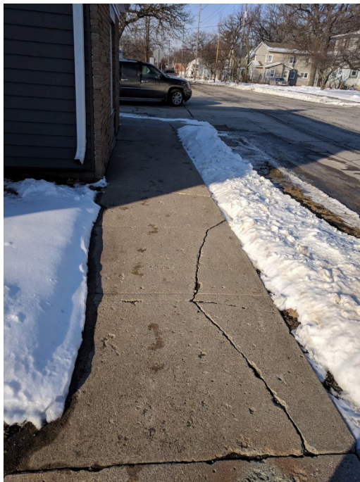
Figure 5. Image of sidewalk requiring replacement.
