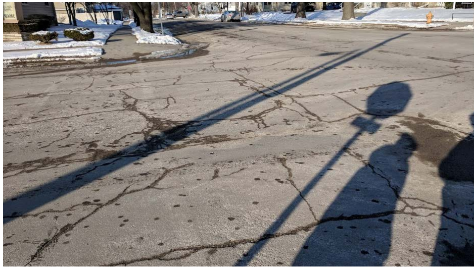
Figure 1. Existing HMA pavement in poor condition
