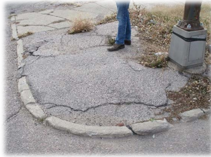
Figure 34 - Example of damaged sidewalks and curbs along Floyd Boulevard. (Photo credit: Rosa Newman, 2014)
