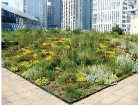
Figure 7. Green roof with various native species on Chicago City Hall. Source: greenroofs.com
