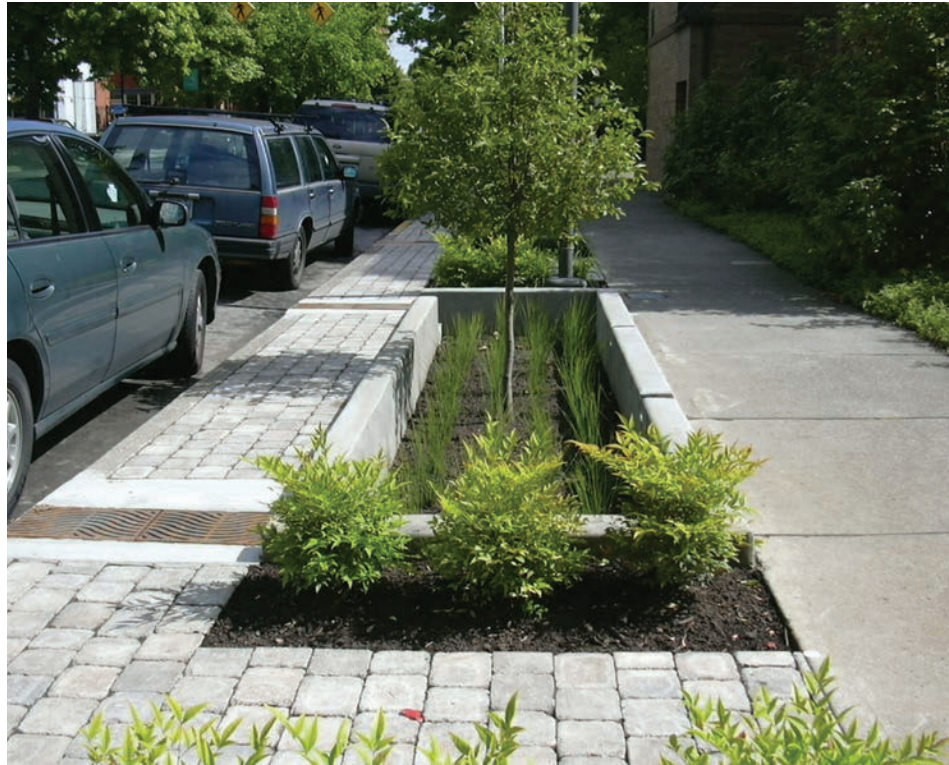
Figure 51. Urban bioswale located in the public right-of-way. Source: Walkable West Palm Beach.
