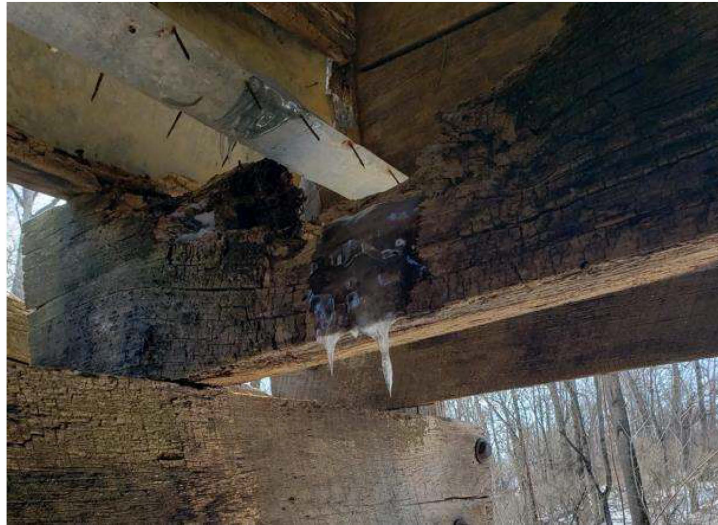
Figure 3.03 – Rotted Members on The Rock Crusher Building
