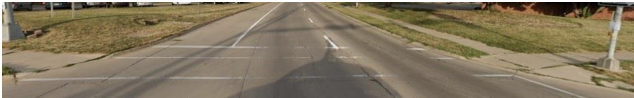
Figure 7: Example of poor conditions of crosswalk
