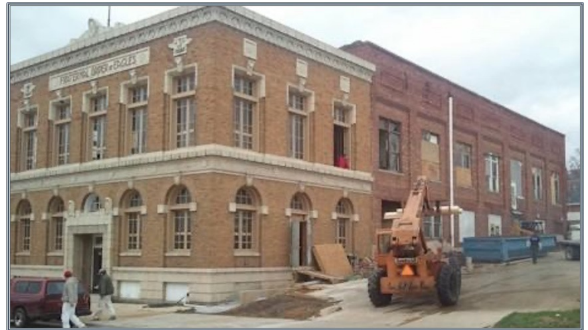
Eagles on Blondeau during construction in 2012. Source: Tri State Public Radio - https://www.tspr.org/post/eagles-building-re-open-january
