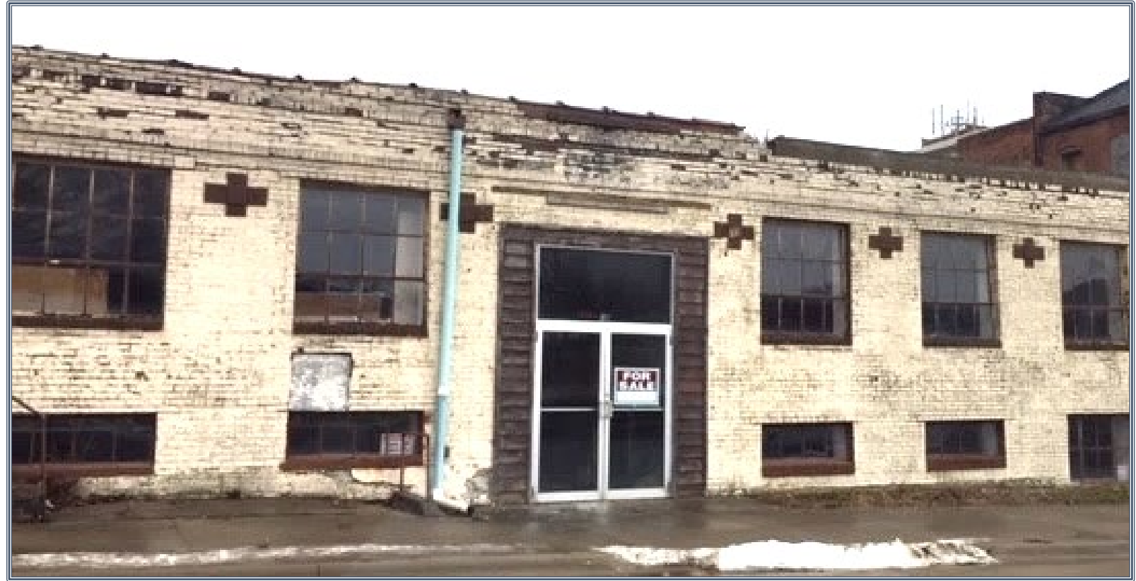
Once home to businesses such as car dealerships and grocery stores, this building at 318 Blondeau Street is an example of the degradation and abandonment that has befallen many downtown commercial structures. Source: Authors.
