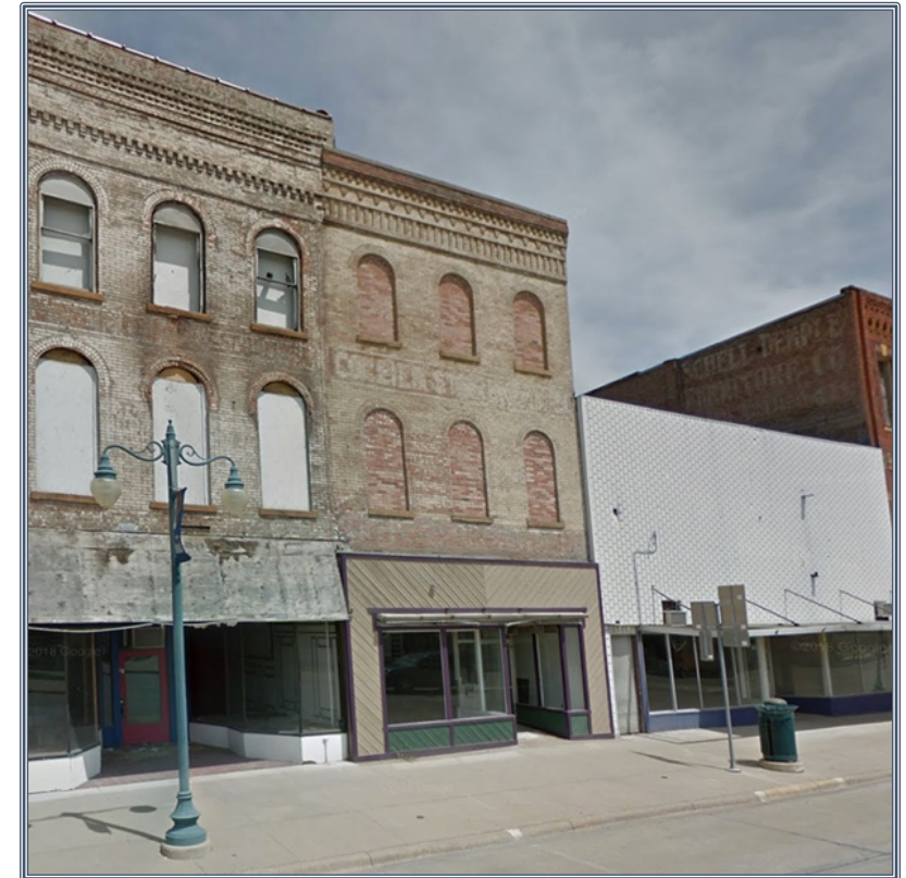
The metal casing on the front of 619 Main Street hides the original façade which appears to still be intact. Source: Google Maps.
