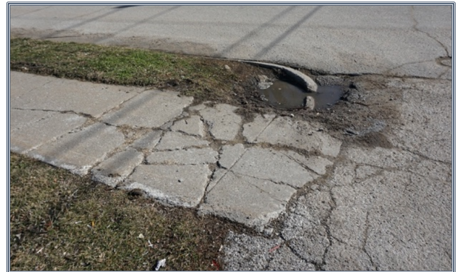
Although this is an alley entrance, repairing the curbing and sidewalk segment would make a sizeable impact on how the entire parcel appears. Source: Authors.
