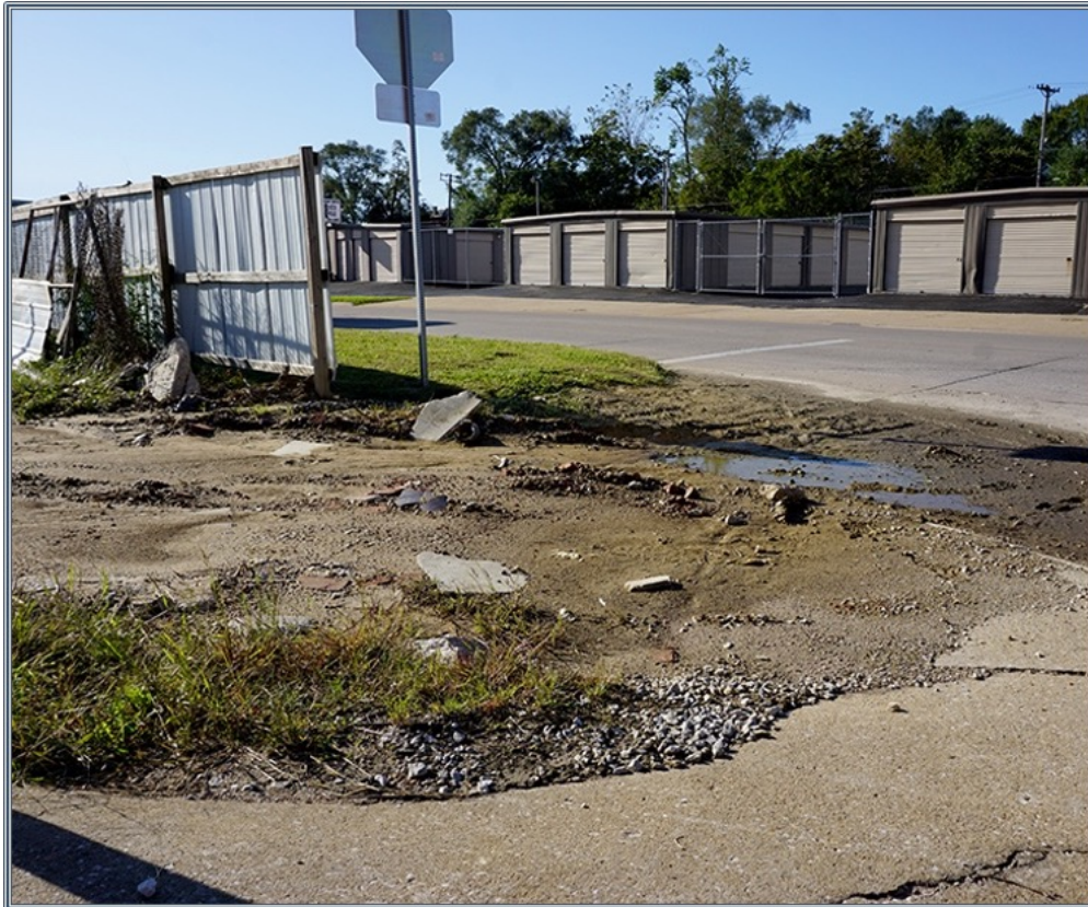
With a lack of accessible sidewalks, large pieces of construction debris, and the stench of a sewer, the corner of Johnson and 7 th Streets presents as a scrapyard rather than a welcoming invitation to the Main Street corridor. Source: Authors.
