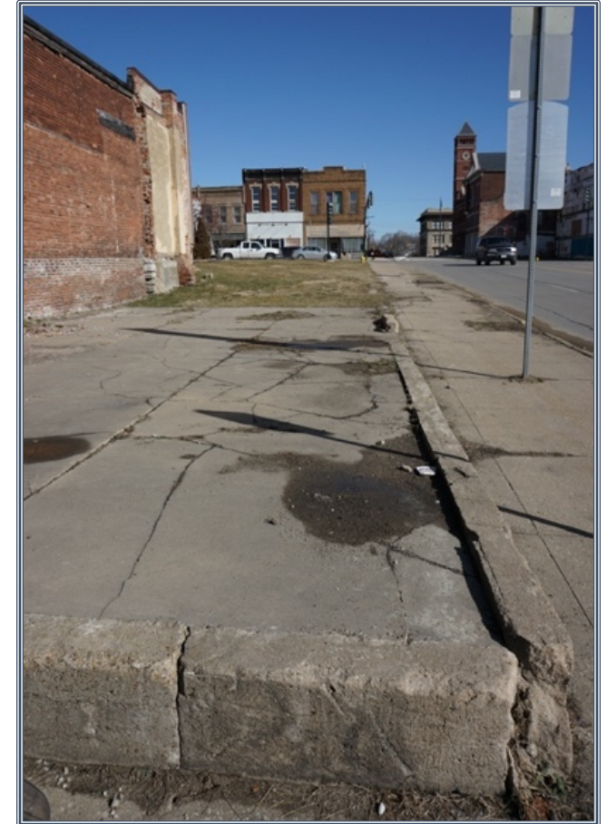
A one-foot high foundation for the none extant news stand is crumbling and unusable for new development. Source: Authors.
