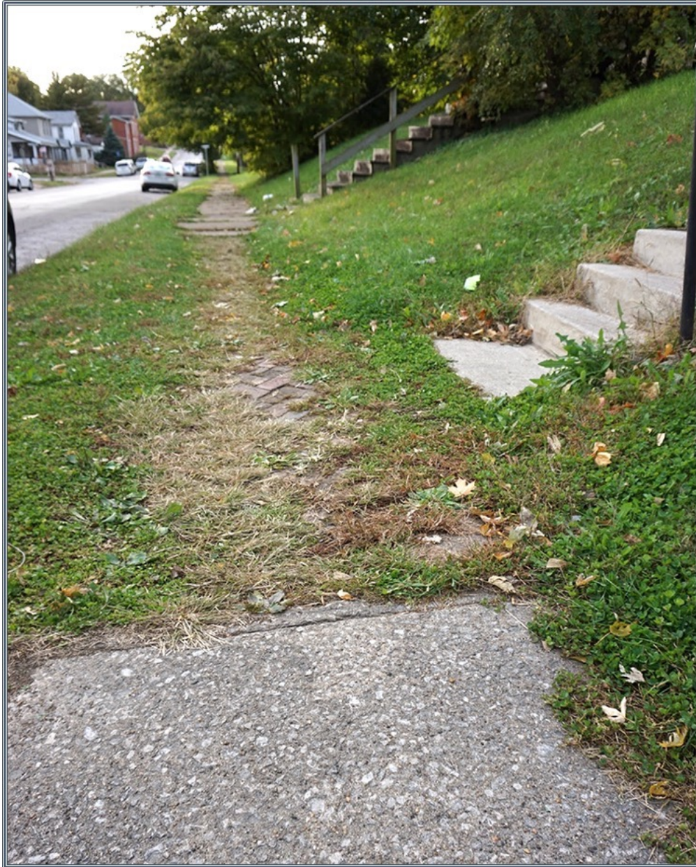
This portion of missing sidewalk on Concert Street is a direct access route for children walking to George Washington Elementary School. Source: Authors.
