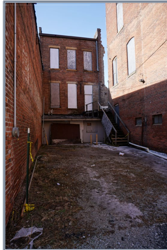
A 2016 fire caused brickwork in the rear of 625 Main Street to crumble. Repairs done in cinder blocks instead of the fallen bricks detracts from the aesthetic appeal of the façade. Source: Authors.
