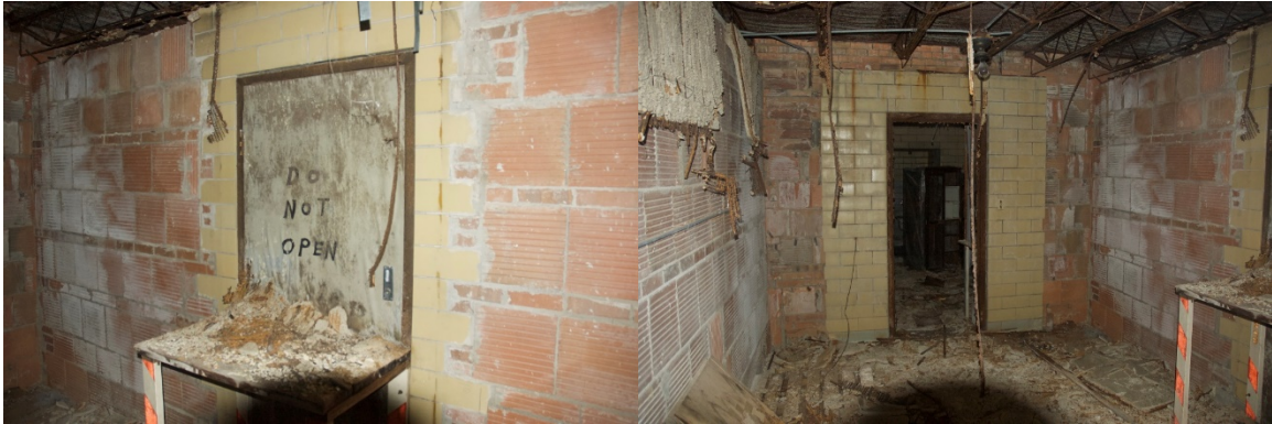
Figure D-1: The ceramic wall tiling was no longer on the wall in most rooms
