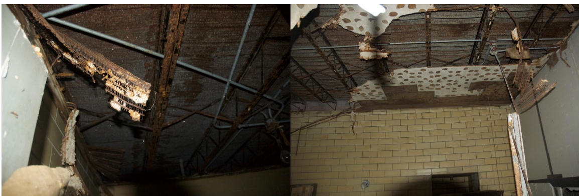
Figure D-2: The roof appeared to have suffered severe water damage. The roofing membrane was severely rusted.
