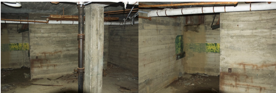
Figure D-4: Foundation of the building appeared to be structurally sound, and in good condition.
