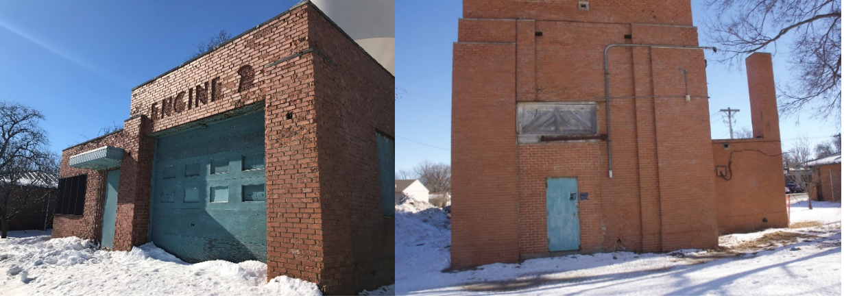
Figure D-5: Exterior of building, the surface of the bricks appeared damaged.
