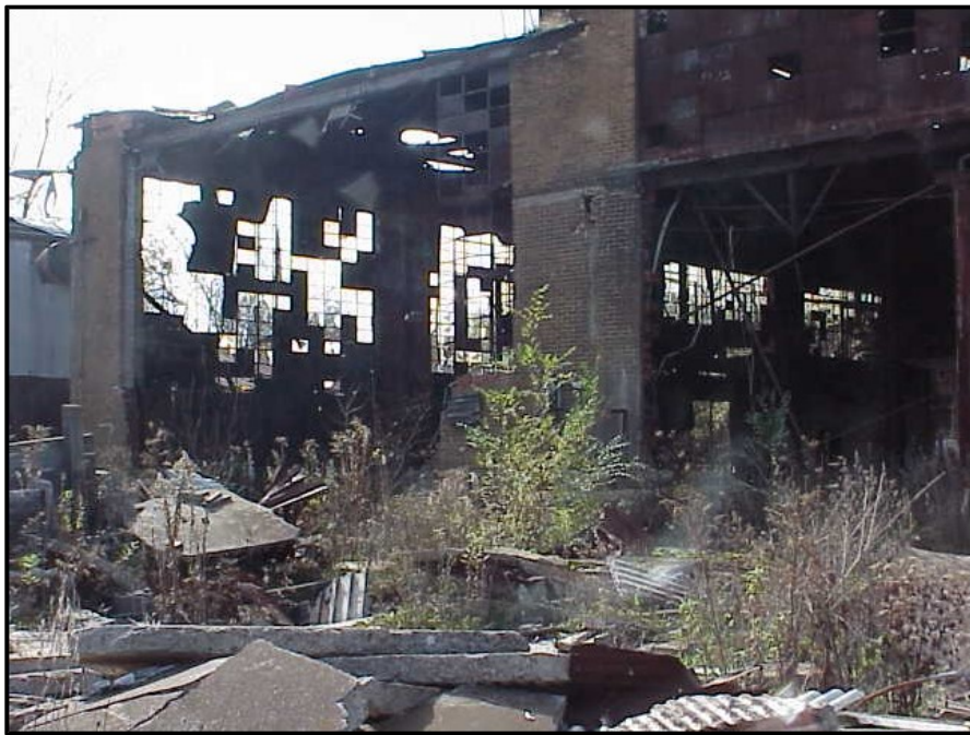
Figure 3.6: A site now remediated in Maquoketa was subject to consistent break-ins. Image source: City of Maquoketa.
