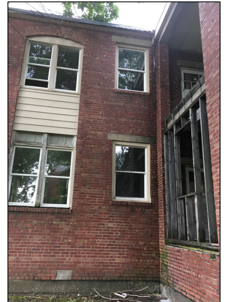
Figure 3.7: Empty buildings at a former army hospital in Clinton have been subject to ongoing criminal activity. Image source: the authors.
